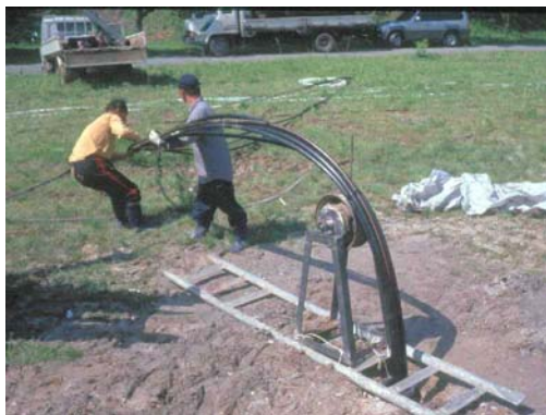
Figure 4: BHE pipe installation in April 2003 using a makeshift roller device (photo Sanner)
