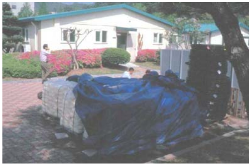
Figure 2: German grouting material and Swiss pre-fabricated BHE on site in Daejon, April 2003 (photo Sanner)
