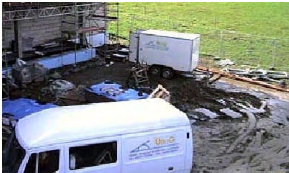
Figure 10: Original UBeG TRT-equipment of UBeG on site for design of a BHE field in Aachen, Germany
