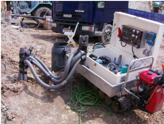
Figure 3: Modern Thermal Response Test rig from UBeG in rough site conditions
