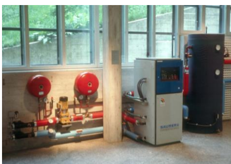
Fig. 9. GSHP in the museum of natural history in St. Gallen, Switzerland (photo from 1993), from [49]
